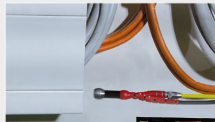
Shafts and underfloor ducting
